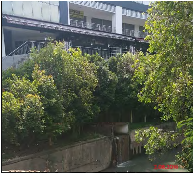
Figure 4.15: Discharge outlet to Station 7
