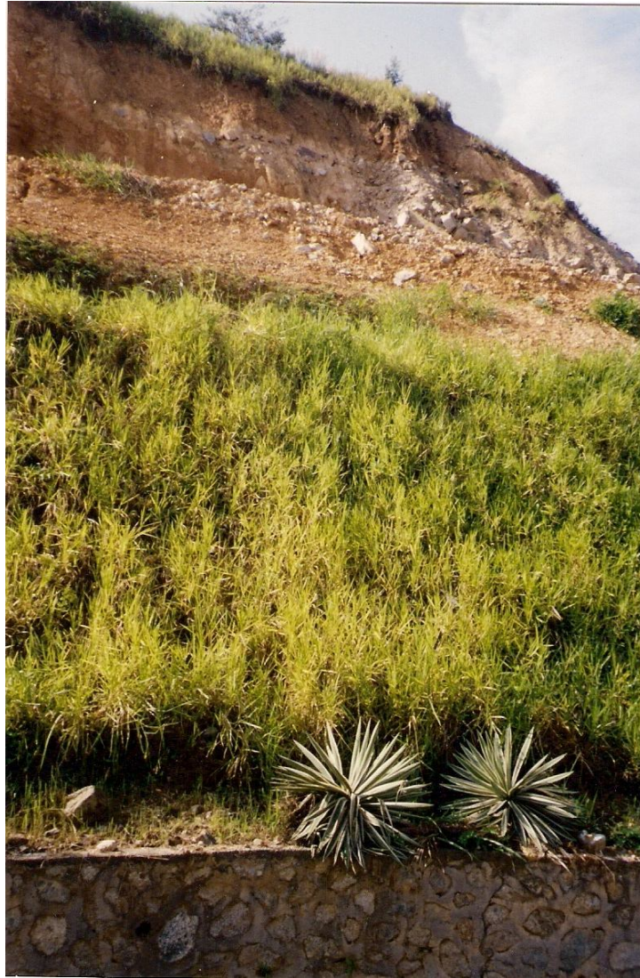
Fig. 4.14: Exposed highly weathered zone with visible relicts of moderately weathered units found in-between.
