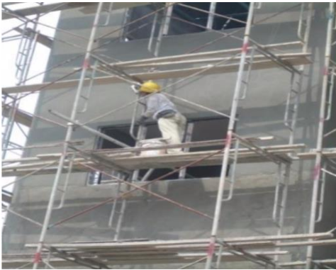
Figure 11: No PPE and No Tag at Scaffolding.
