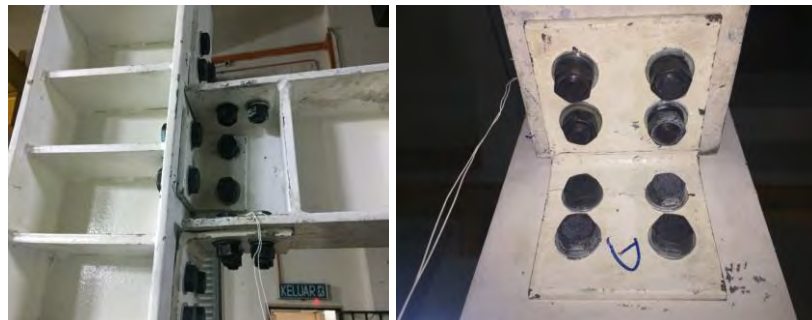
Figure 5.11: Failure pattern of the angles in the bare semi-rigid frame (zoom view)
