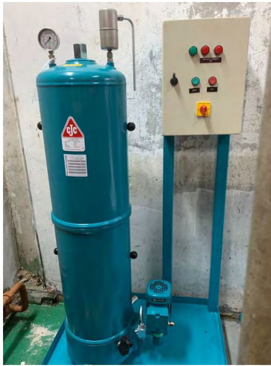
Figure 3.3: CJCT TM HDU 27/108 Fine Filter at site
