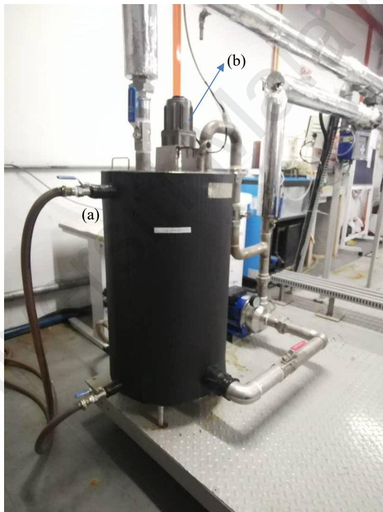
Figure 3.7: (a) Reservoir tank (b) Agitator motor
