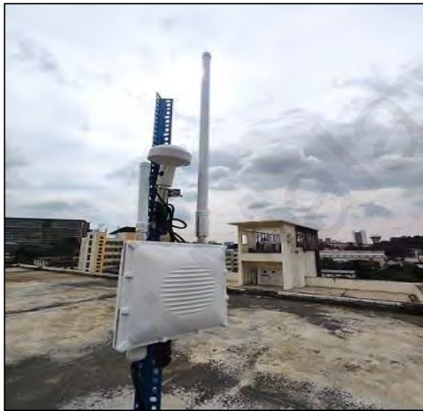
Figure 3.6: LoRa Gateway on Top of the Roof
