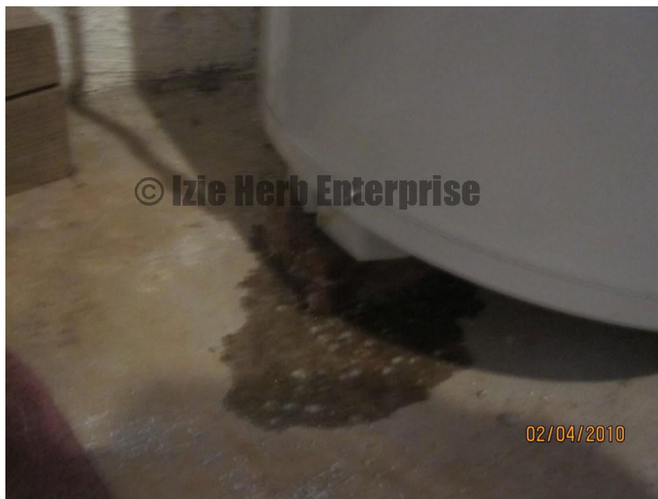
Figure 4.7: Spillage of water below the rinse area
