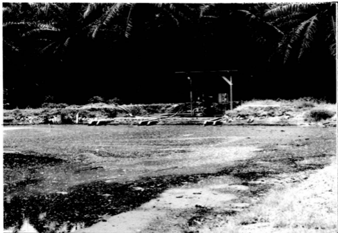
EFFLUENT TREATMENT POND WITH PUMPSET
