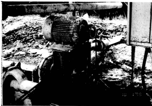
CLOSE UP VIEW OF CORRODED PUMPSET AND BASE FRAME
