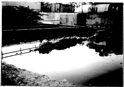
CORROSION OF EFFLUENT BASIN
