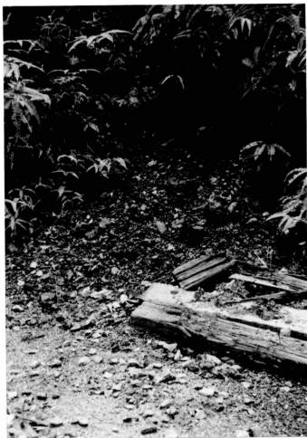
Plate 3.3 Weathered graphitic schist exposed on embankment along the railway line (Location : ST 3 – 5km from Mambau)
