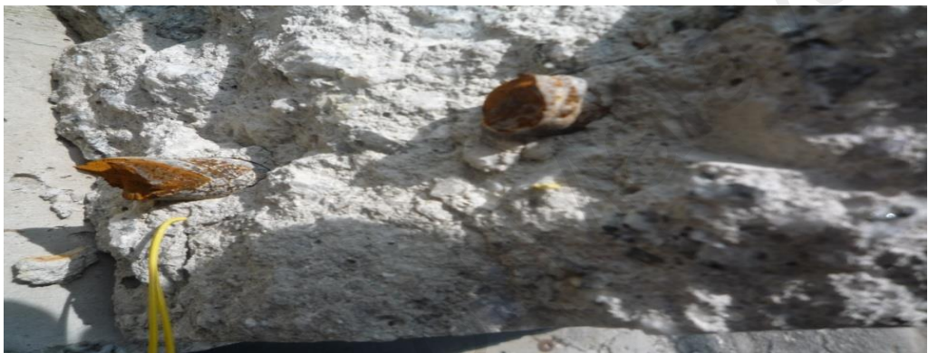
Figure 4.57: Fatigue fracture of steel
