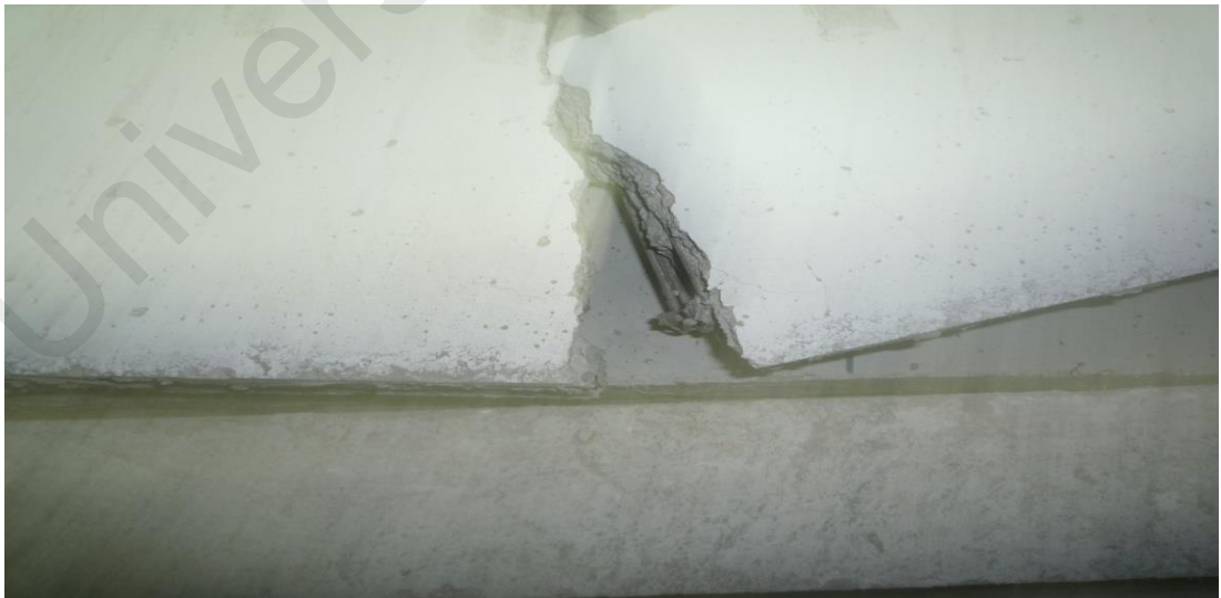
Figure 4.58: Failure mode of NSF
