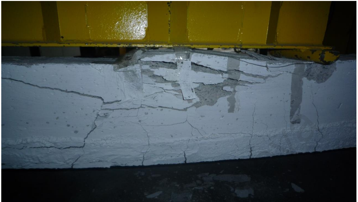
Figure 4.44: Failure mode of N2SS8C
