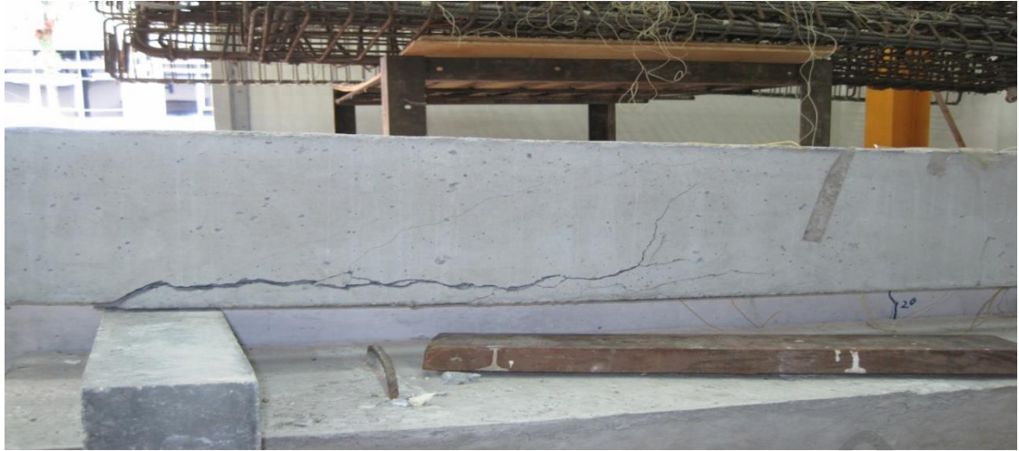
Figure 4.6: Debonding failure mode of H2B6S19L73W2.76T
