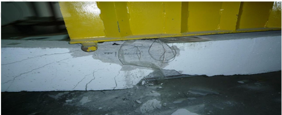
Figure 4.43: Failure mode of N1SH8C
