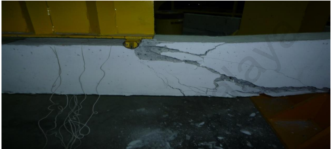
Figure 4.1: Debonding failure mode of H1B8S19L73W2T
