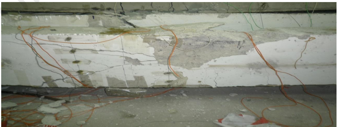
Figure 4.11: Flexure failure mode of H1B8S19L73W2TAF
