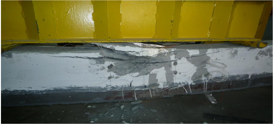
Figure 4.12: Flexure failure mode of SH2B6S19L100W2T
