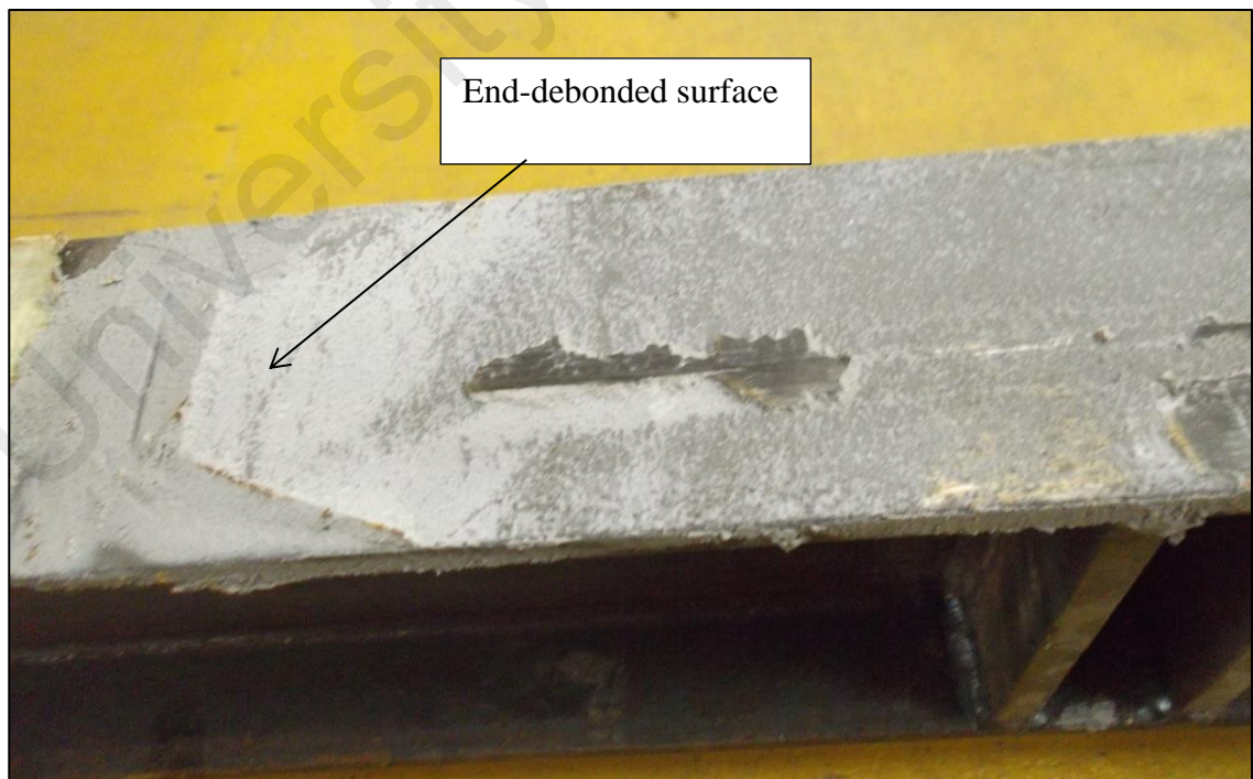
Figure 4.7: CFRP end debonded steel surface
