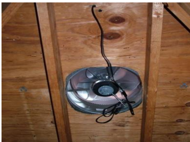
Figure 2.10: Attic fan (Carter, 2016).
