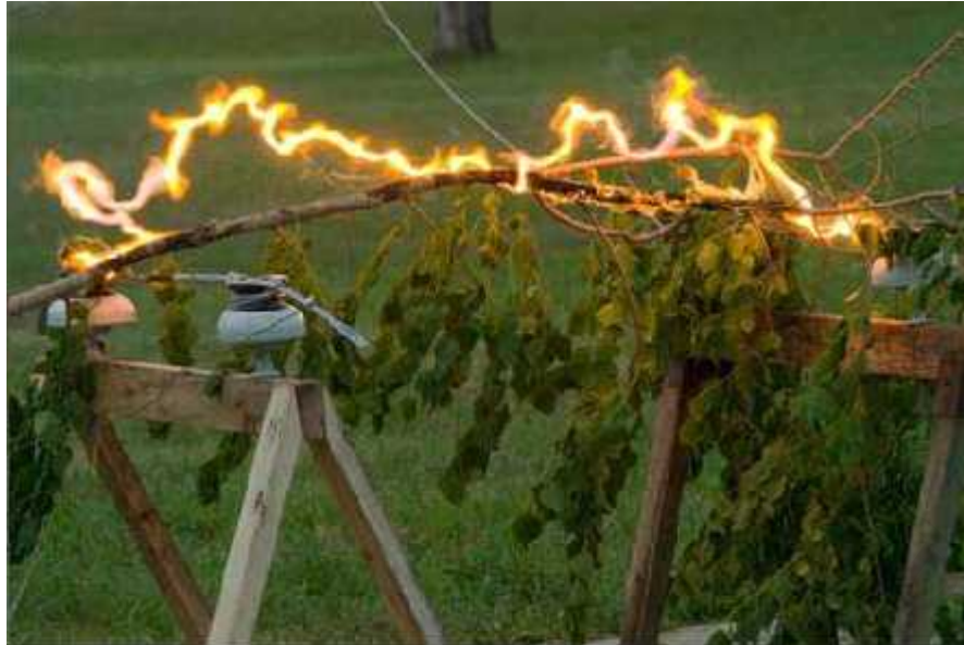
Figure 3.3 : An electric arcing phenomenon
