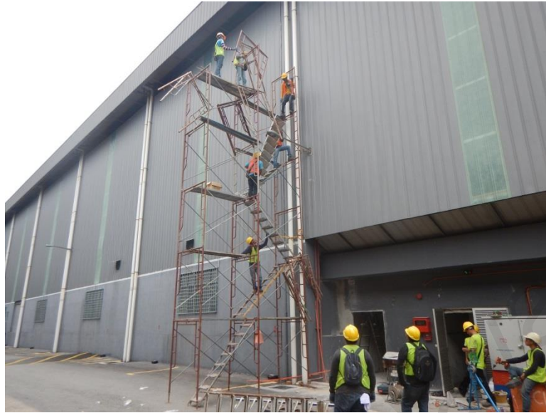
Figure 4.5: Workers were installing the scaffolding as the main access to the rooftop
