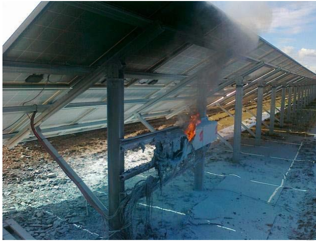
Figure 2.4: A fire in a connection box in a ground PV system. (Ref. [25])
