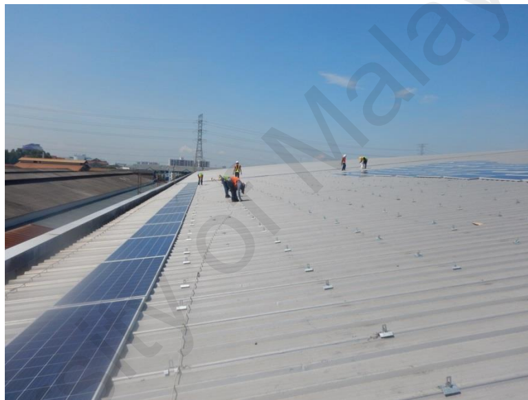
Figure 4.8: Workers were installing the solar PV brackets on the rooftop under sunny day
