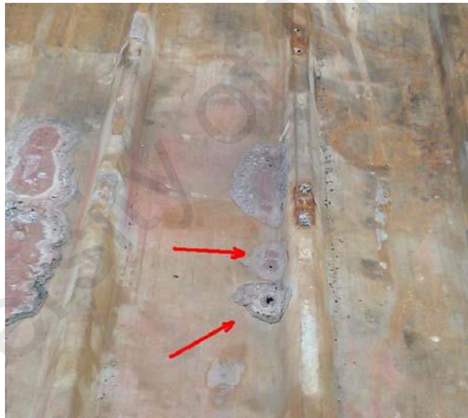
Figure 2.5: DC arcing effects on an external side of polyurethane (Ref. [25])
