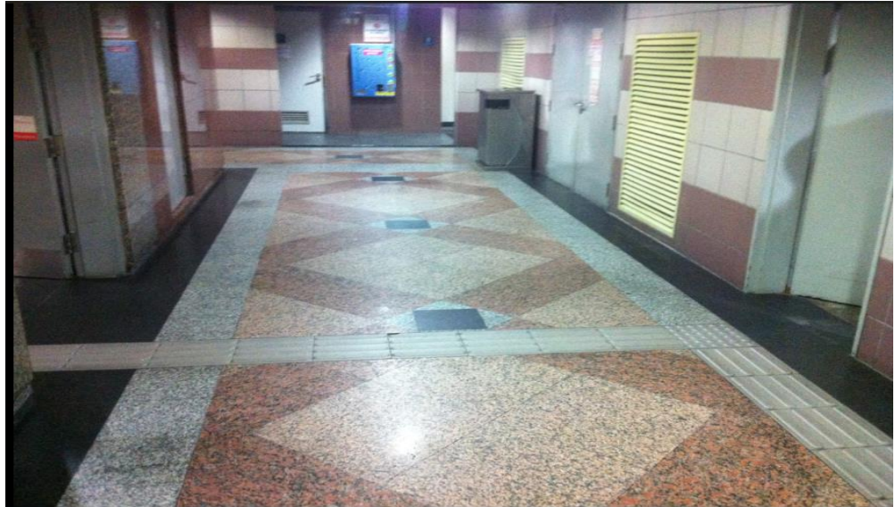
Figure 3.4(b) incomplete disabled Lavatory (toilet) pedestrian route.
