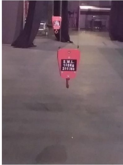
Figure 4.10: Dangling counterweights during stage set up at Pentas 1, Kuala Lumpur Performing Arts Centre, KLPAC
