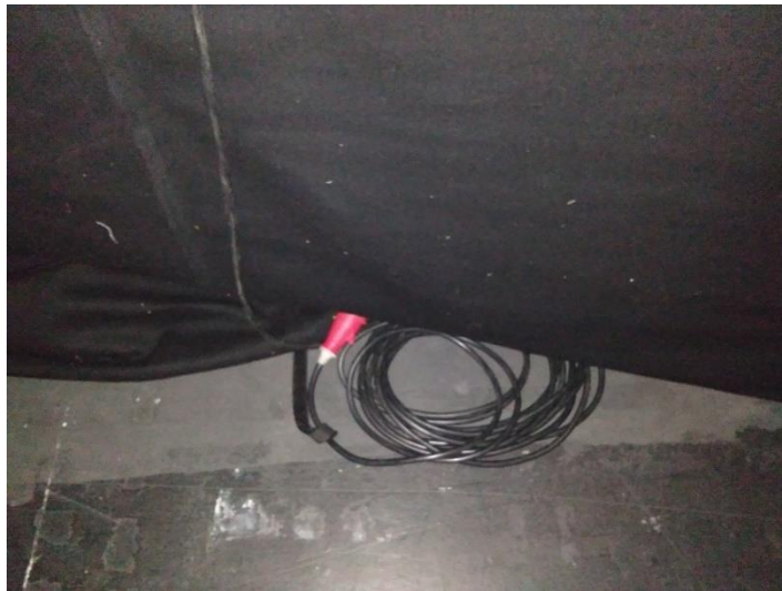
Figure 4.25: Wiring on the ground backstage at Pentas 1, Kuala Lumpur Performing Arts Centre, KLPAC
