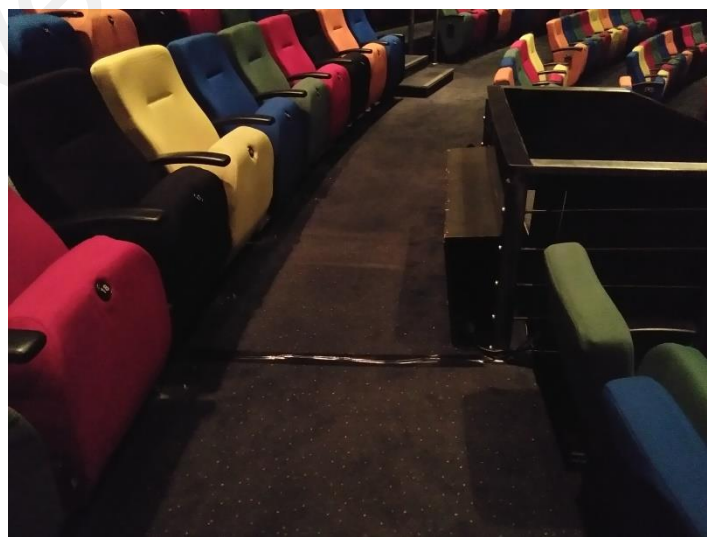
Figure 4.29: Tripping hazard at Pentas 1, Kuala Lumpur Performing Arts Centre
