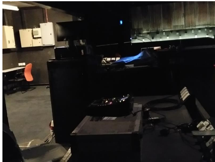
Figure 4.20: Technical Control Area at Pentas 1, Kuala Lumpur Performing Arts Centre
