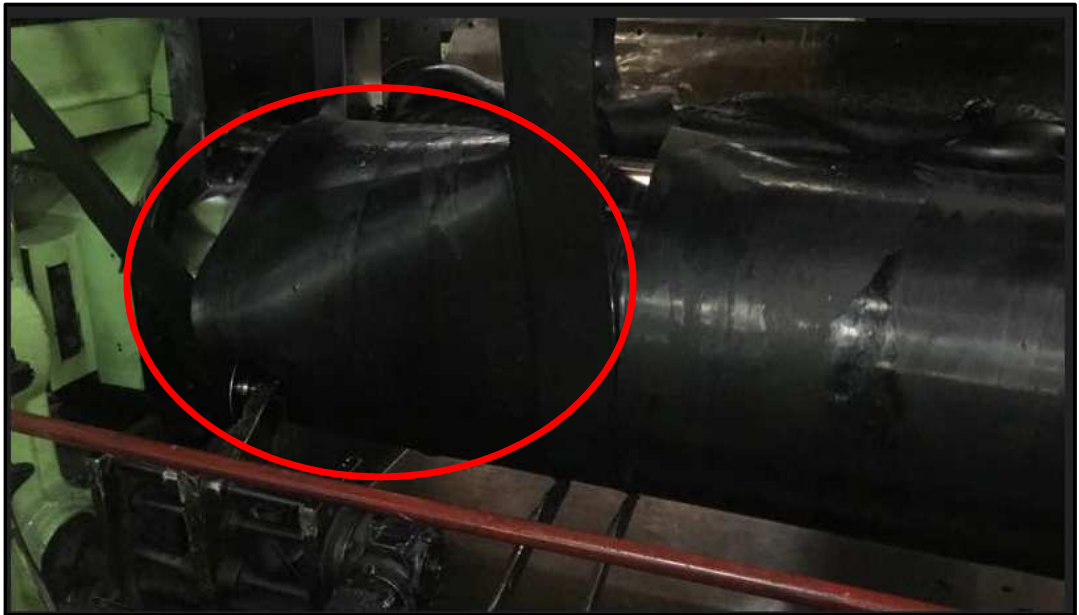
Figure 5.1 Looping issue in cracker mill due to high mooney viscosity
